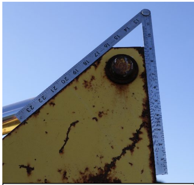
To measure an angle using the Line of Chords, first set the leaves of the rule to match the angle to be measured. In this case, a steel plate.
