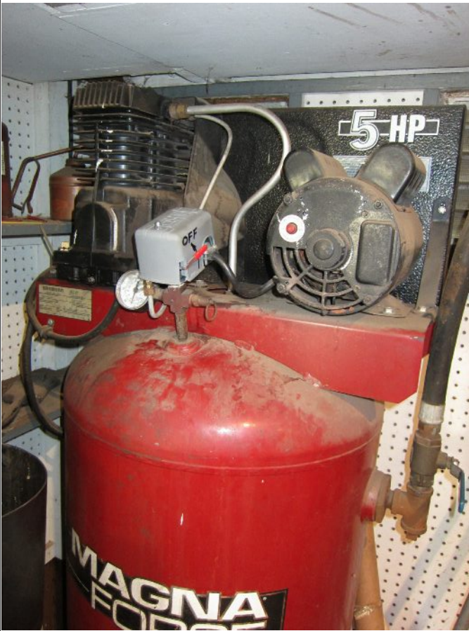
Photo 1: The Air Compressor Setup
