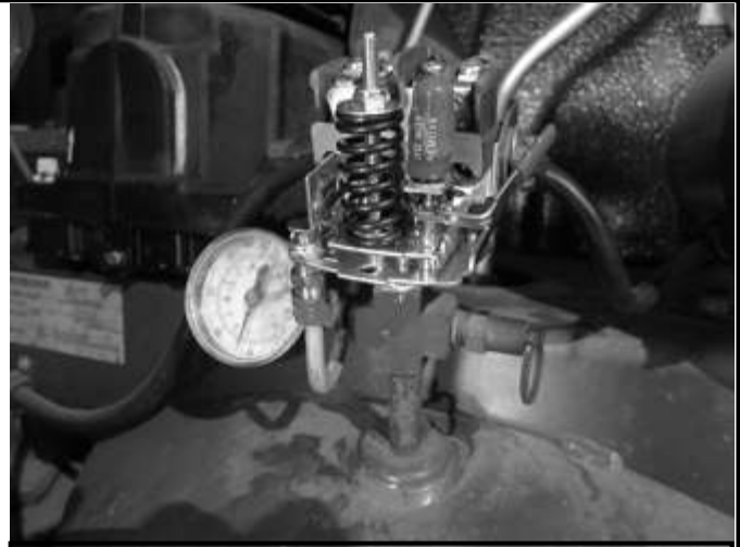
Photo 2: The Pressure Switch
