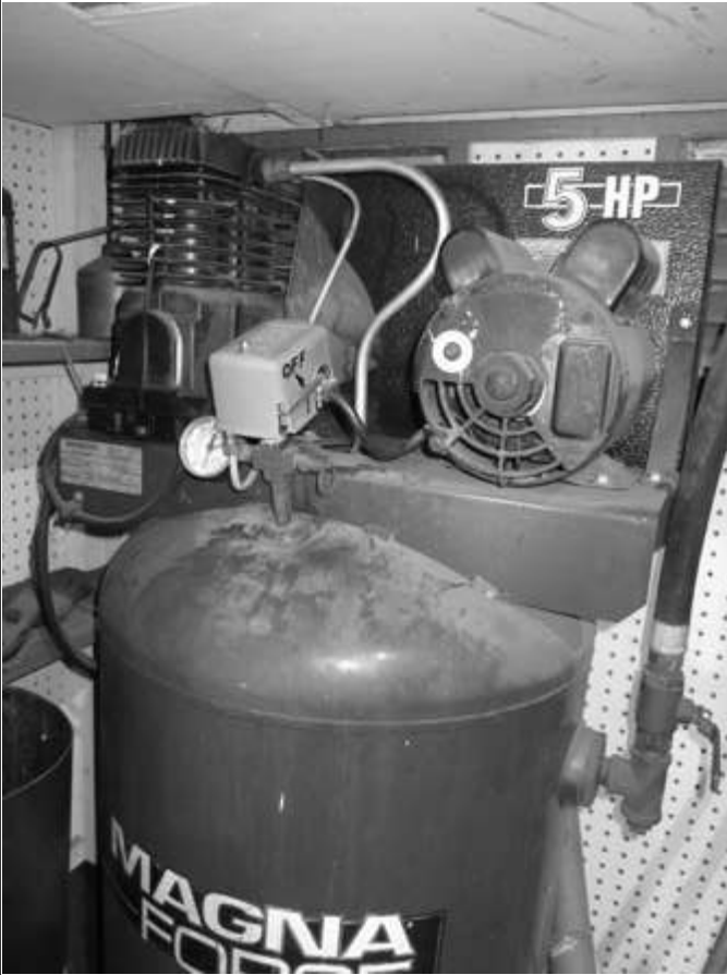
Photo 1: The Air Compressor Setup
